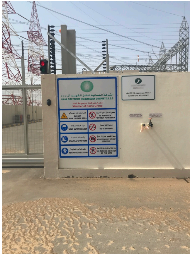
Figure 2-10 Entrance to Constructed Substation (July 2019)
