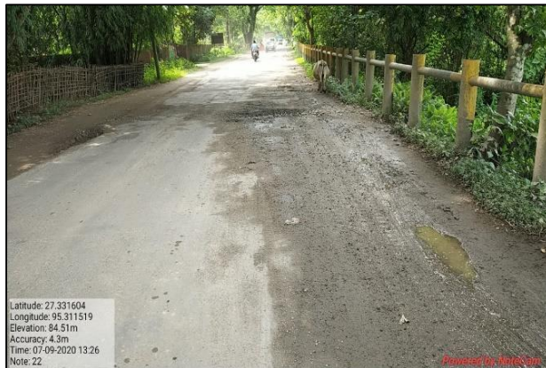
Exhibit-3: Road Condition
