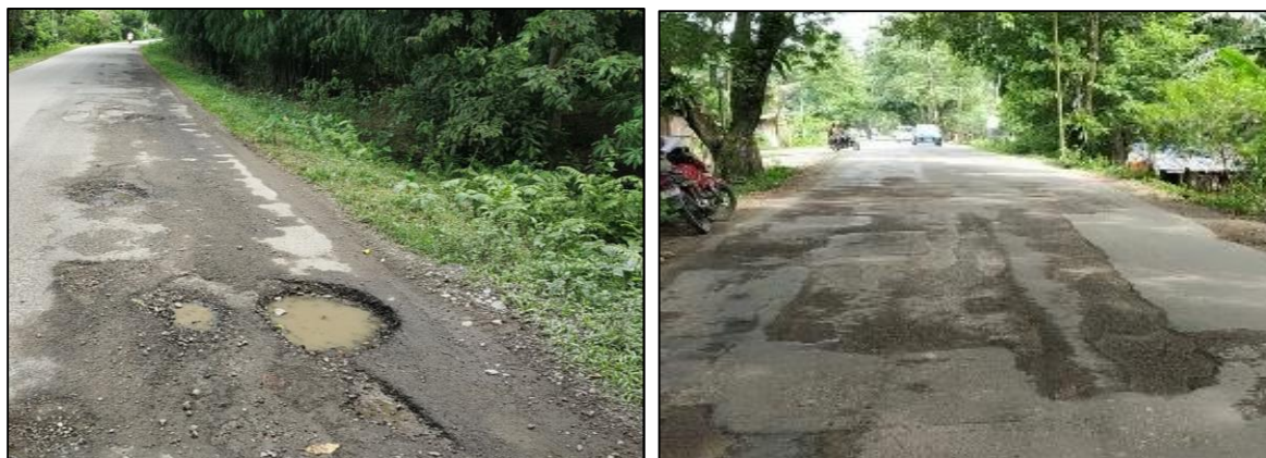
Figure 1- 3: Photo of highly distressed road along stretch
