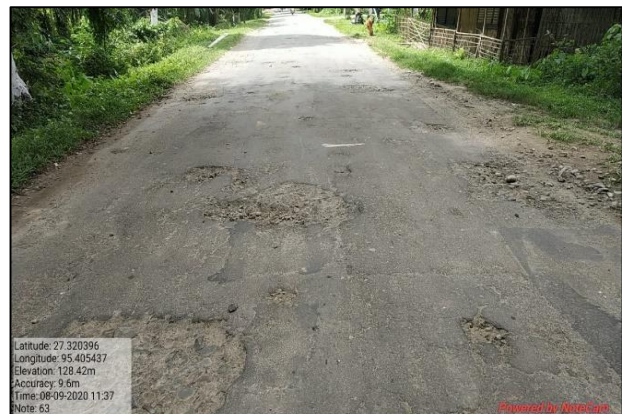
Exhibit-4: Road Condition
