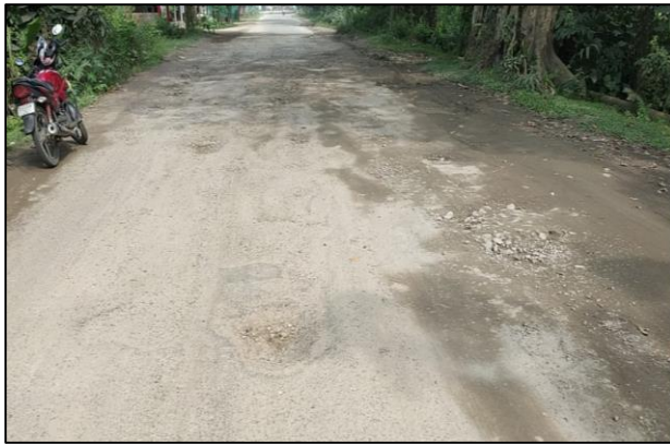
Exhibit-1: Road Condition
