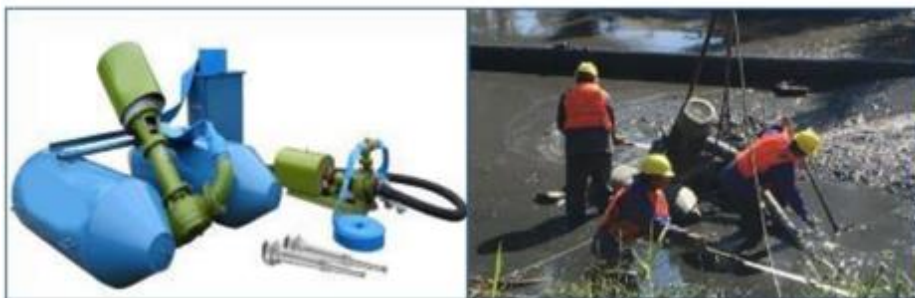
High concentration sludge pump
