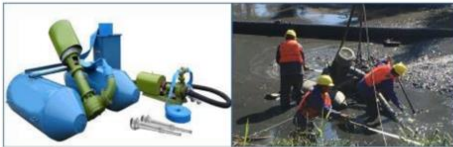
High-concentration sludge pump
