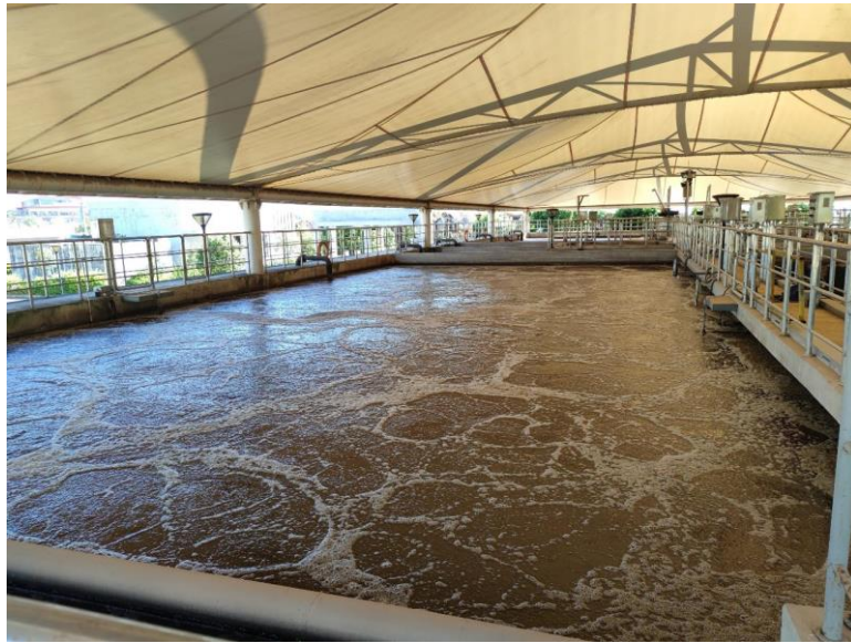
Fig. 1 Wastewater treatment system
