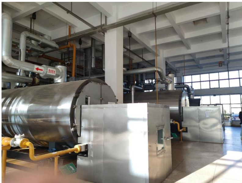
Fig. 10 Gas Boilers at Power Energy Center
