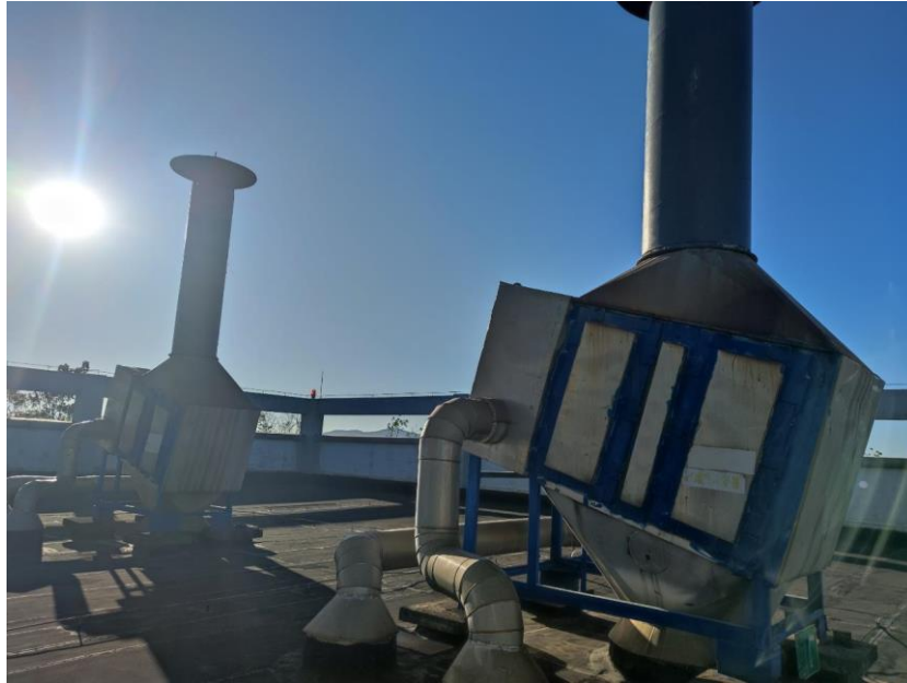
Fig. 11 Gas boiler stack
