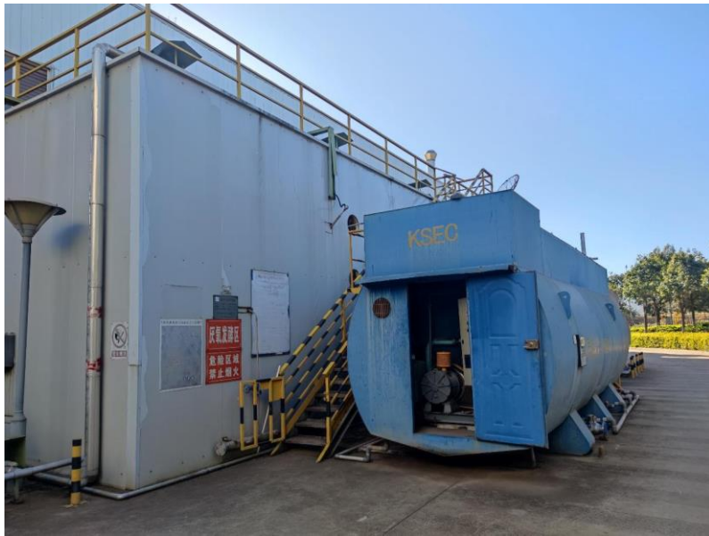
Fig. 7 Domestic waste leachate treatment device
