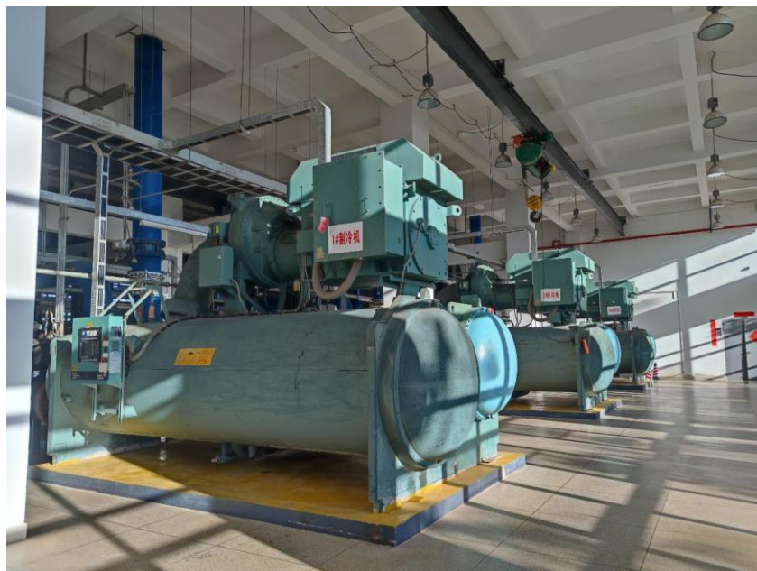
Fig. 12 Chiller units at the Power and Energy Center
