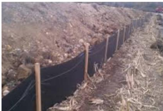
Figure 6 - Silt fence installed around soil storage stockpiles to prevent soil erosion and excessive sedimentation with stormwater runoff.
