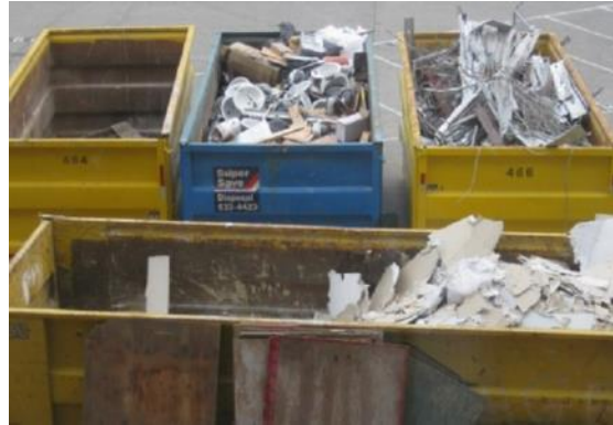
Figure 5 - Construction waste will be segregated and temporarily collected on-site for further proper disposal/recycling off-site.
