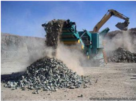
Figure 4 - Dust generation during construction works.
