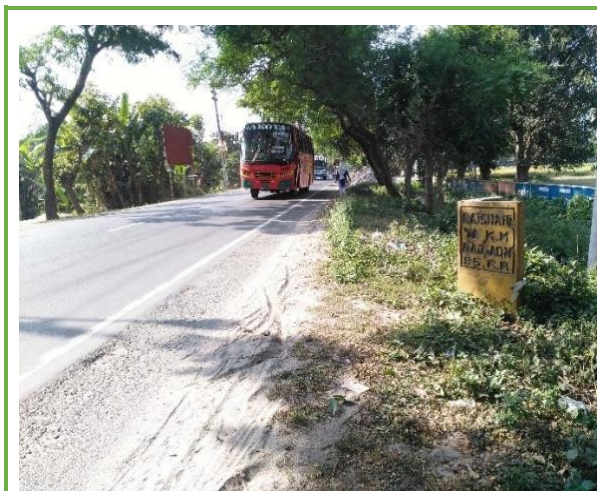
Figure 4.41 Broken letters of milestone of roadside
