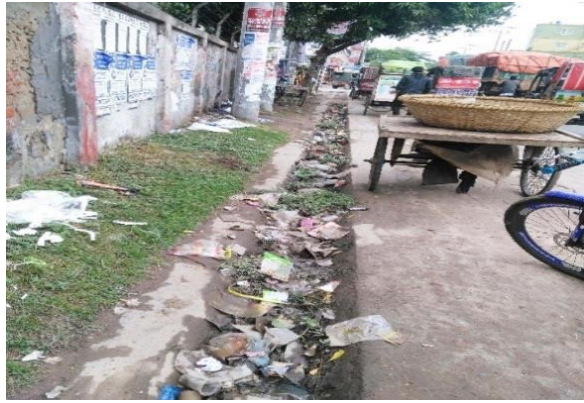
Figure 4.43 Blocked drain at Kajla, Rajshahi
