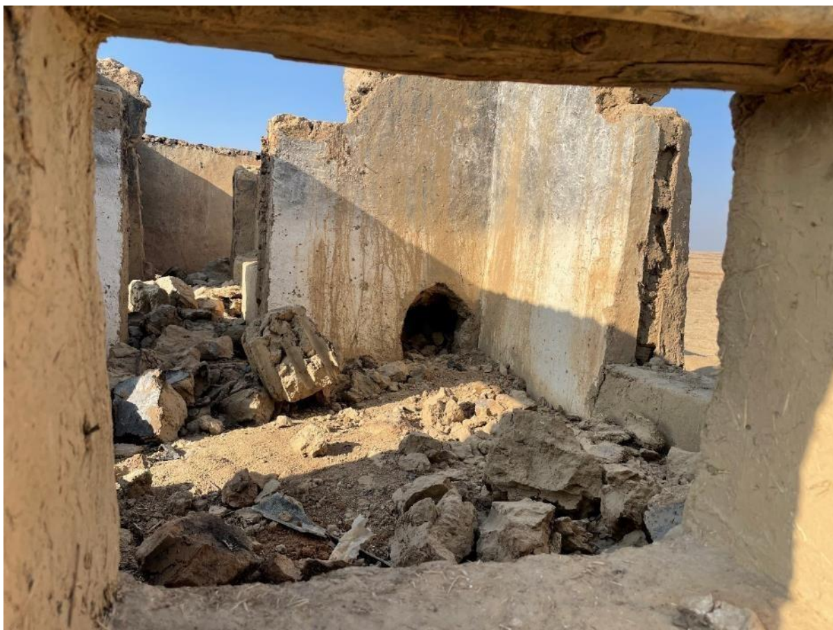
Figure 6-40. Inside of ruined Farm 5 house
