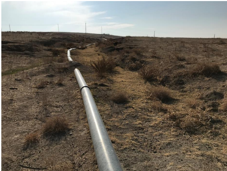
Figure 6-16. Water pipe from Zarafshan River (west of site)
