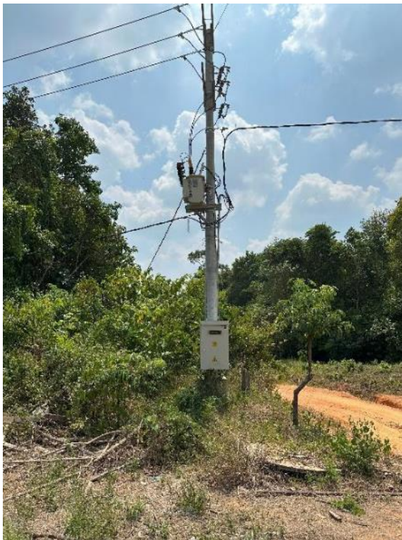
Electricity Substation in the Village Electricity Project in UID S2JB.
