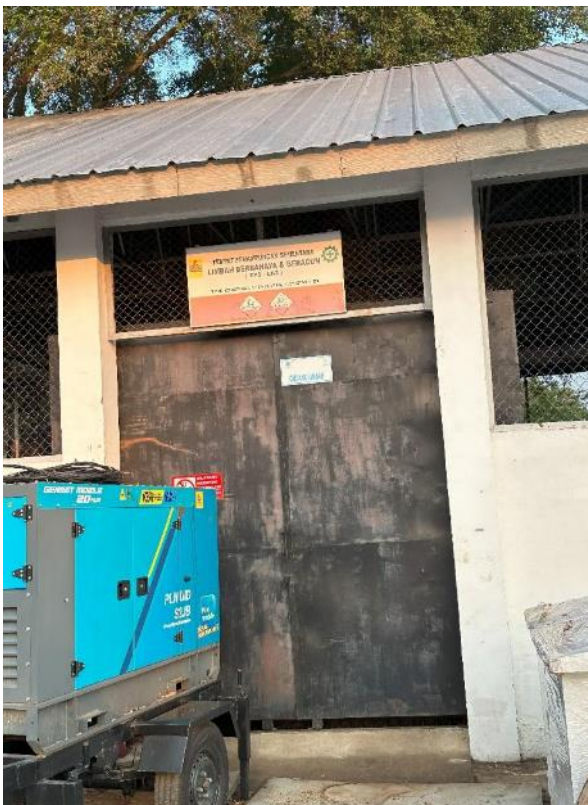
Temporary storage of hazardous waste (B3) in the Keramasan Warehouse in UID S2JB.
