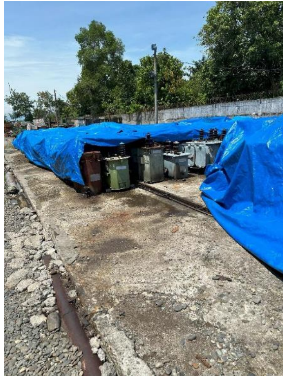
Used transformer storage outside and some do not have a lid in Binjai warehouse in UID North Sumatra.
