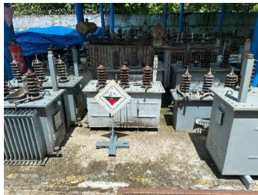
Inappropriate symbol labeling of used transformer in Binjai warehouse in UID North Sumatra.
