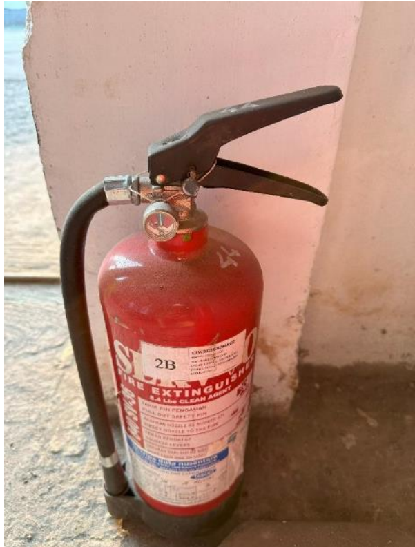
Low pressure extinguisher in the Keramasan Warehouse in UID S2JB.
