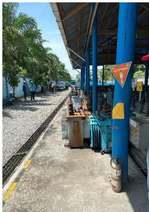
Placement of transformers that have been and have not been drained outside the area where there is a spill collection channel in Binjai warehouse in UID North Sumatra.
