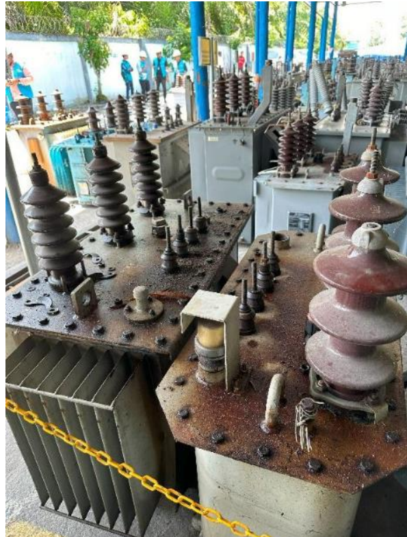
Used transformers with oil spills on the top are stored in Binjai warehouse in UID North Sumatra.
