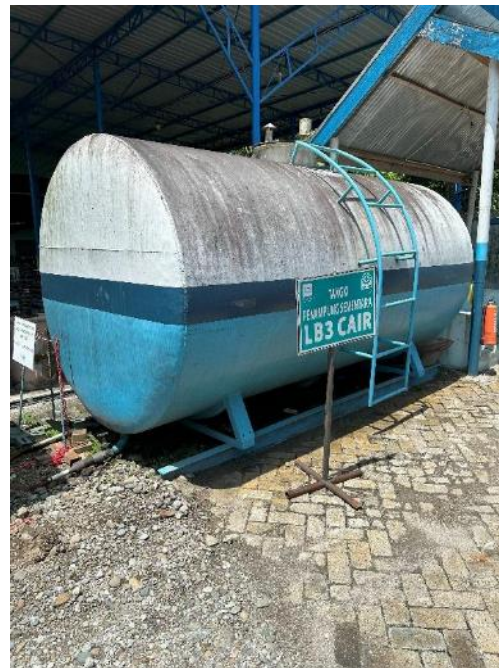
The tank for waste transformer oil has no containment near the temporary storage of hazardous waste in Binjai warehouse in UID North Sumatra.
