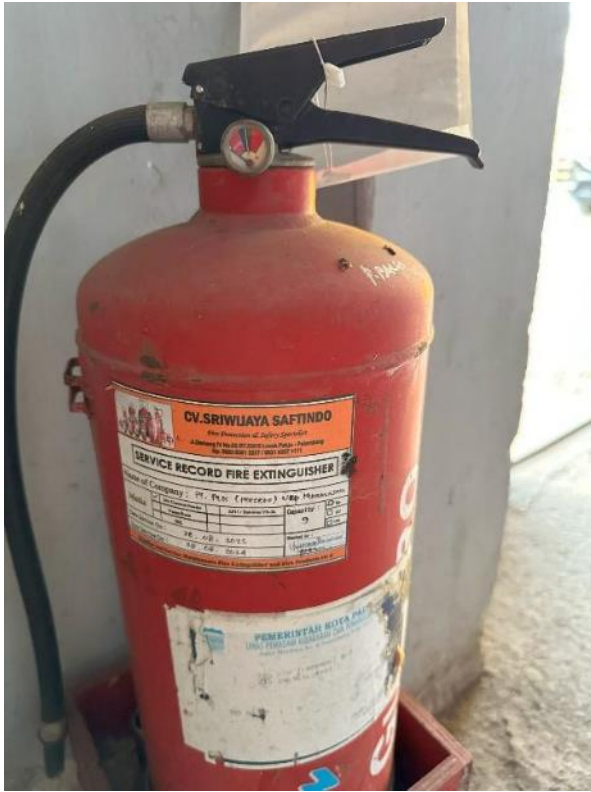
Expiring and no pressure extinguisher in the Keramasan Warehouse in UID S2JB.
