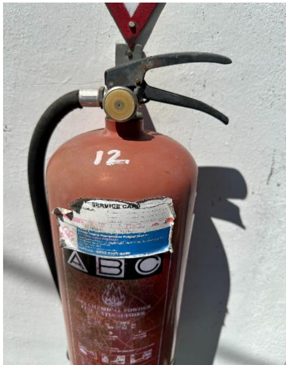
Expired fire extinguisher in Banda Aceh warehouse in UID Aceh.
