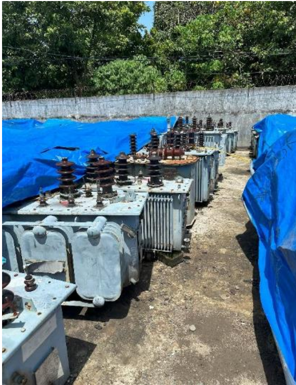
Used transformer storage outside and some do not have a lid in Binjai warehouse in UID North Sumatra.
