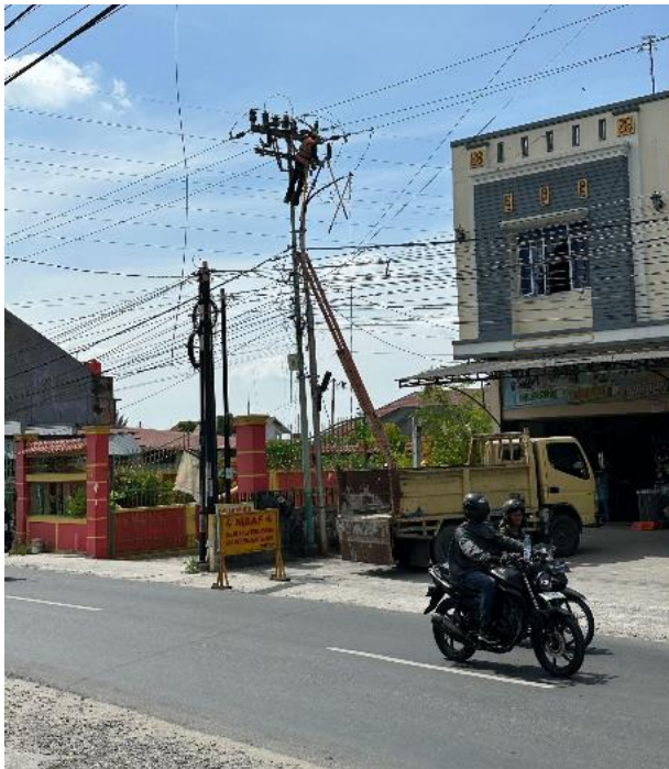
Working at height without barricade during installation of lightning arrester in UID RKR.
