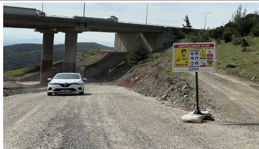
Figure 95. Information and warning signs in the activity area of Başpınar Viaduct
