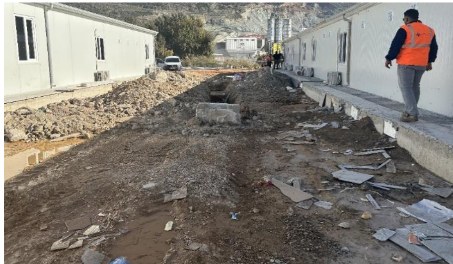
Figure 68. Hazardous Conditions in Kuruyer Construction and Accommodation Area
