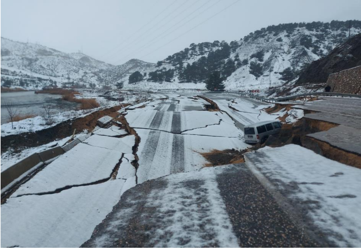
Figure 18. Damage on the Transformers Zone (Malatya-Gölbası Road KM:89+260-KM:30+100)
