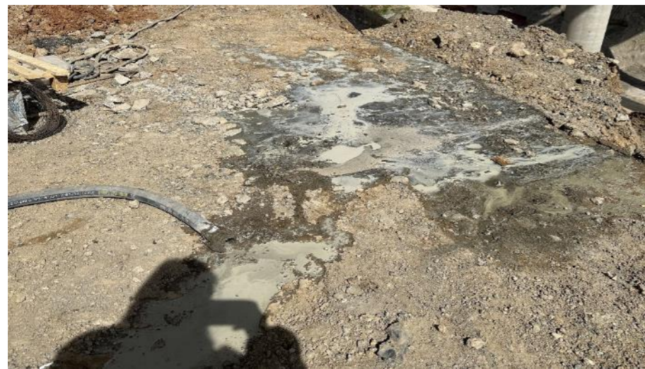
Figure 92. Soil Contamination in the activity area of Başpınar Viaduct
