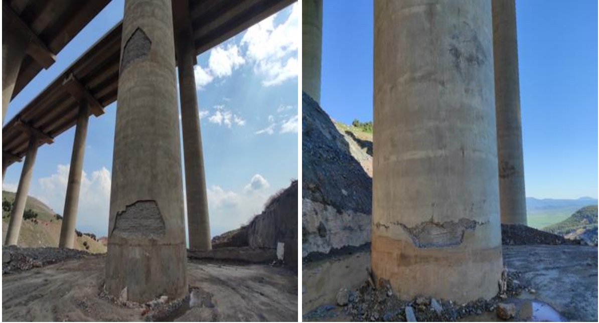
Figure 5. Damages on the Piers – Şehitler Viaduct
