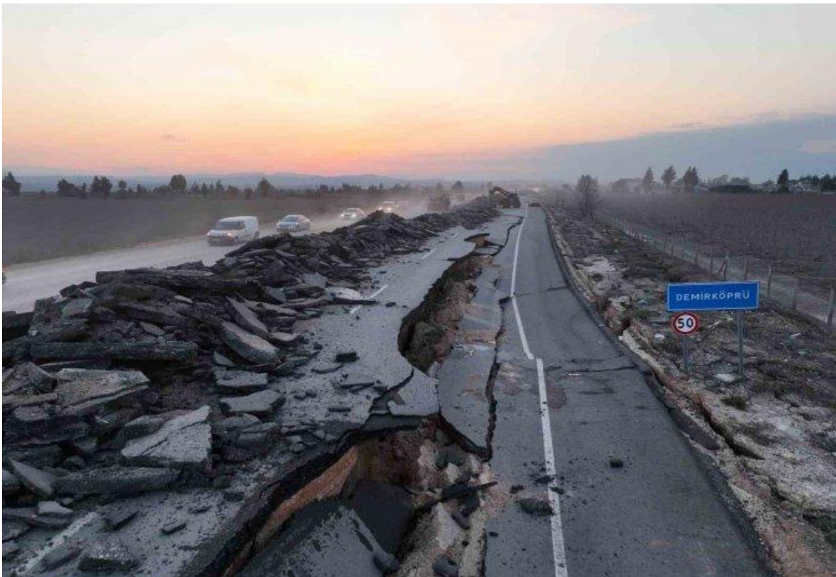
Figure 11. View of the Demirköprü Bridge After the Earthquake
