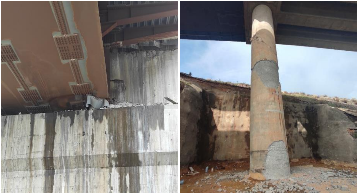
Figure 6. Damages on the Nurdağı Viaduct
