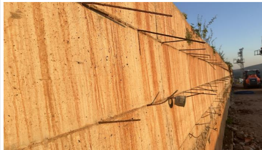
Figure 51. Hazardous Behaviors at the Kızılkaya Construction and Accommodation Site-1
