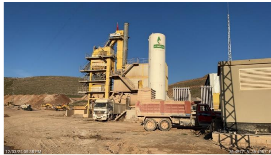
Figure 39. Asphalt Plant in Kizilkaya Quarry
