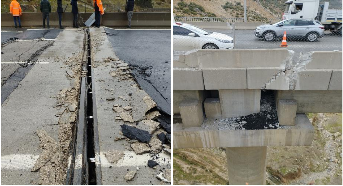
Figure 7. Damages on the Başpınar Viaduct
