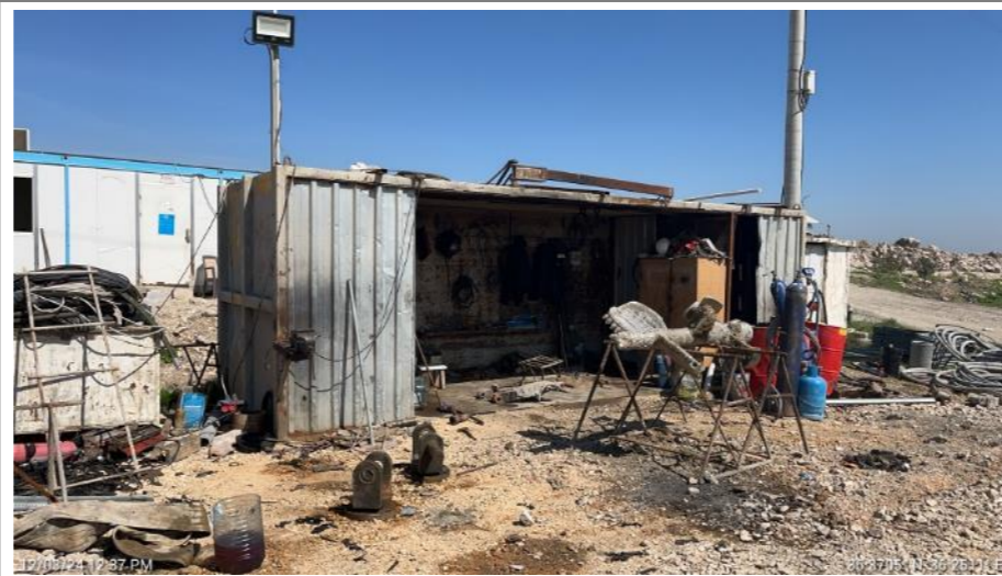
Figure 45. Poor Management of Wastes and Chemicals-1 at the Hatay Airport Road
