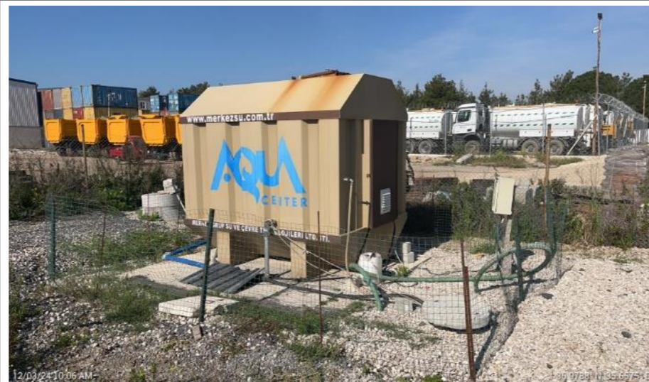
Figure 84. Package WWTP in Ceyhan Construction and Accommodation Site
