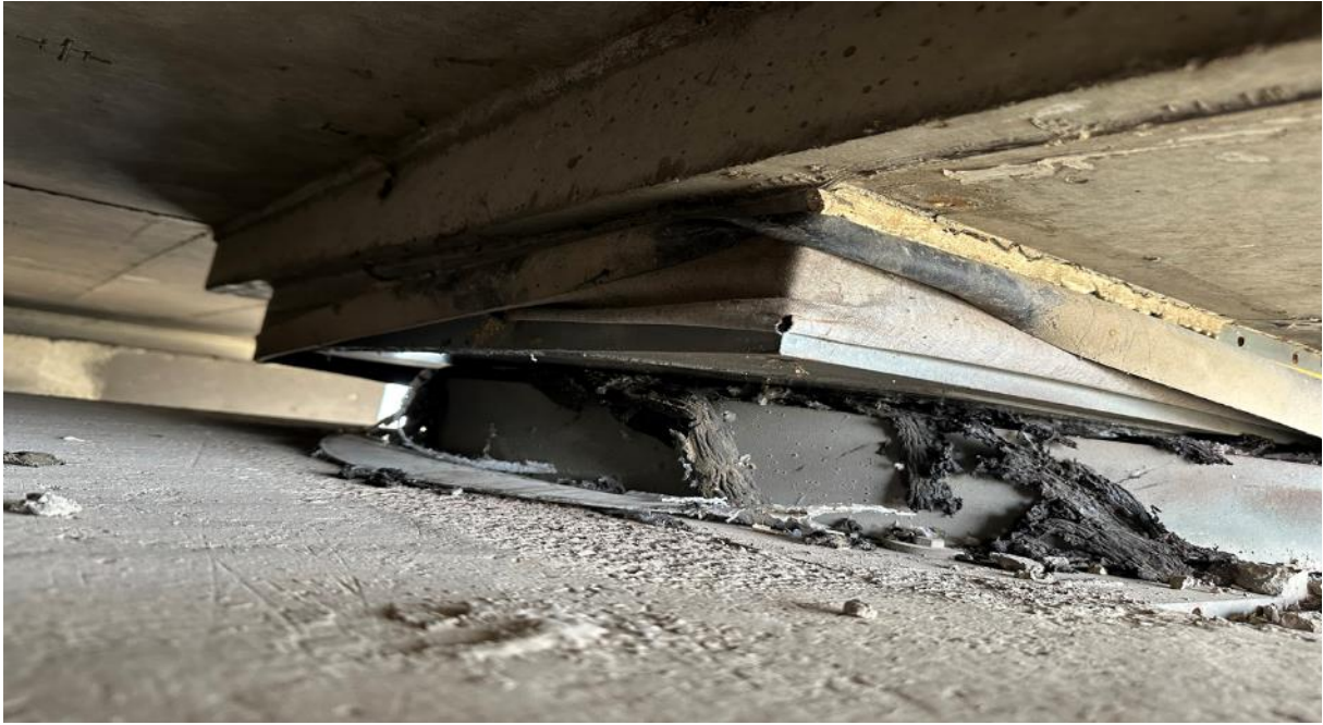
Figure 24. Damages on the Structural Bearings
