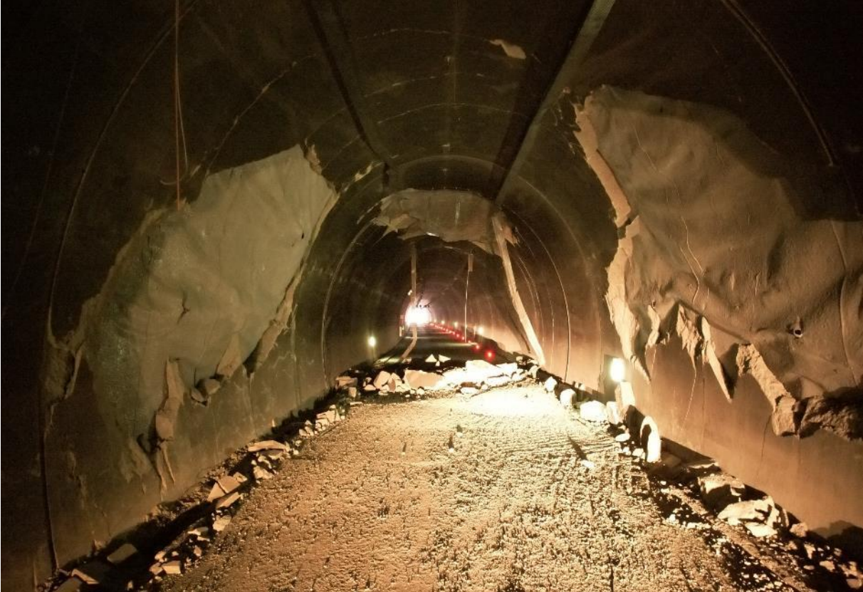
Figure 19. Damage on Erkenek Tunnel Entrance Portal Area
