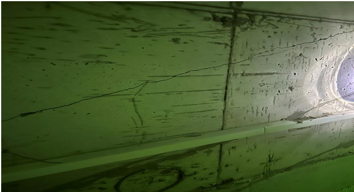
Figure 23. Hairline Shear Cracks
