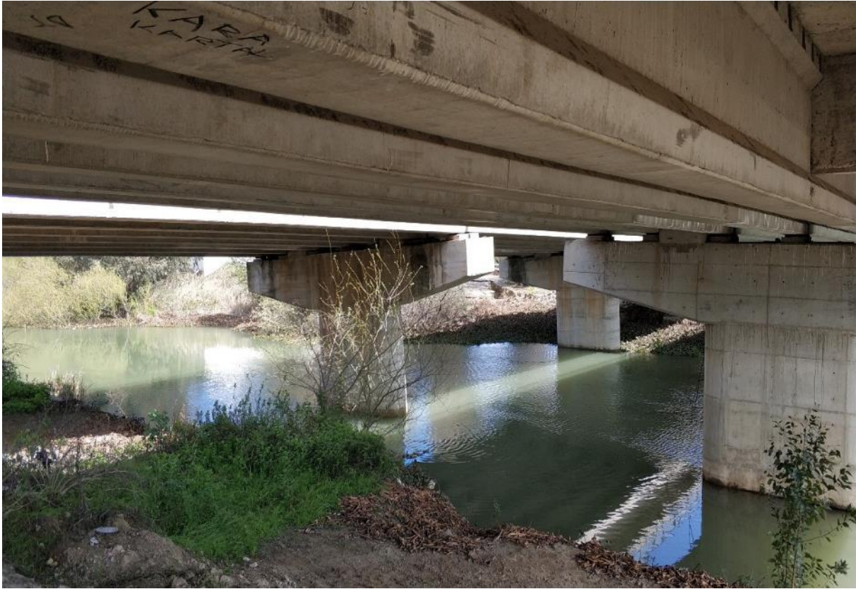
Figure 10. Damage on the Bridge Piers
