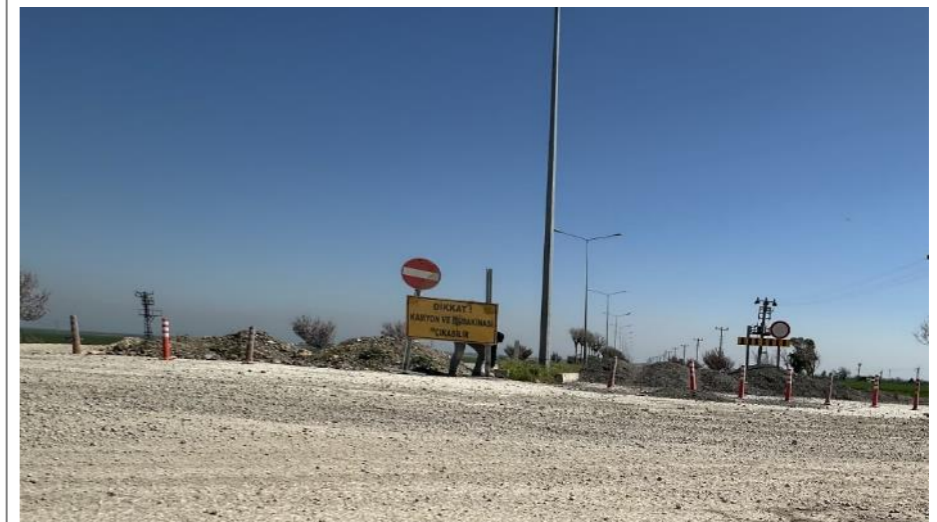
Figure 49. Warning Sign at the Hatay Airport Road Construction Site
