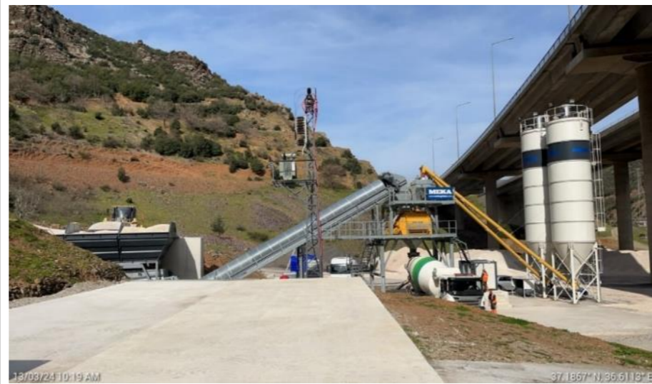
Figure 81. Bahçe (Ayran) Concrete Plant
