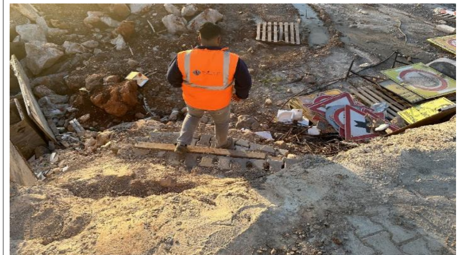
Figure 52. Environmental and OHS Non-conformity at the Kızılkaya Construction and Accommodation Site-2
