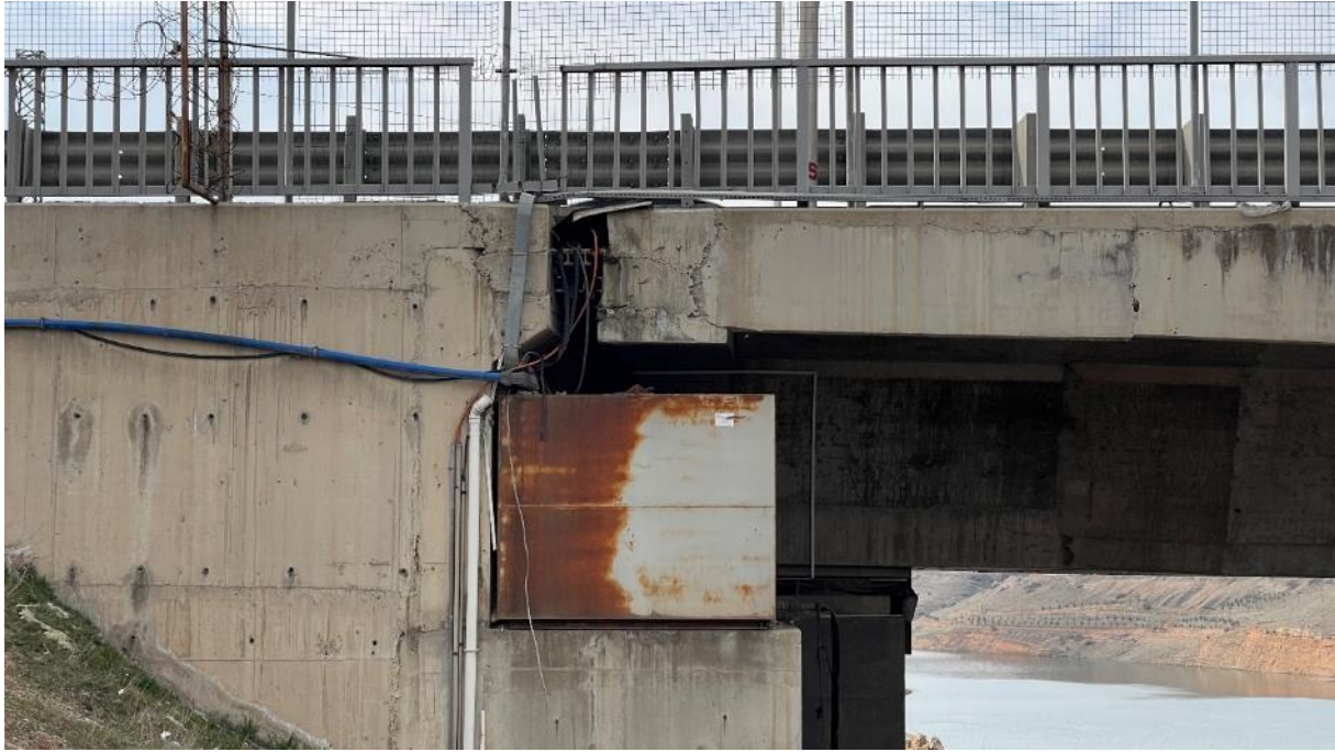
Figure 99. Damages on the Bridge
