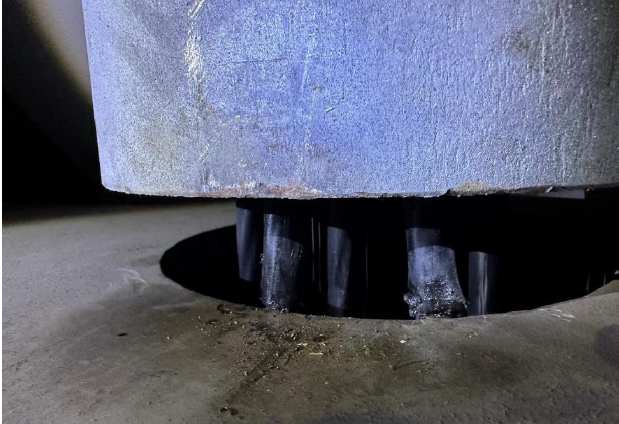
Figure 29. Damaged Suspension Cables
