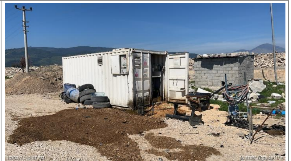
Figure 46. Poor Management of Wastes and Chemicals-2 at the Hatay Airport Road
