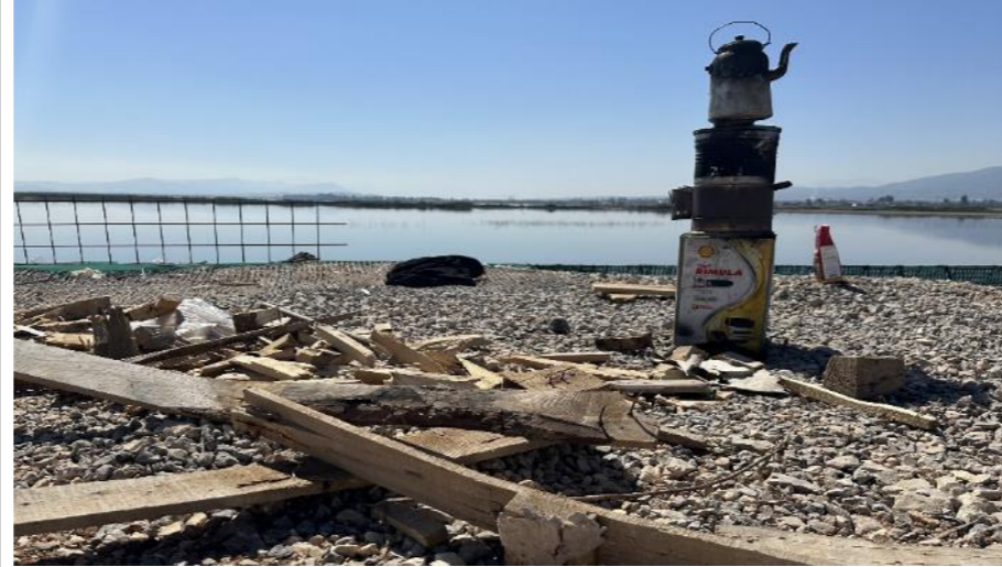
Figure 54. Hazardous Conditions and Hazardous behavior at the Hatay Airport Road Construction Site
