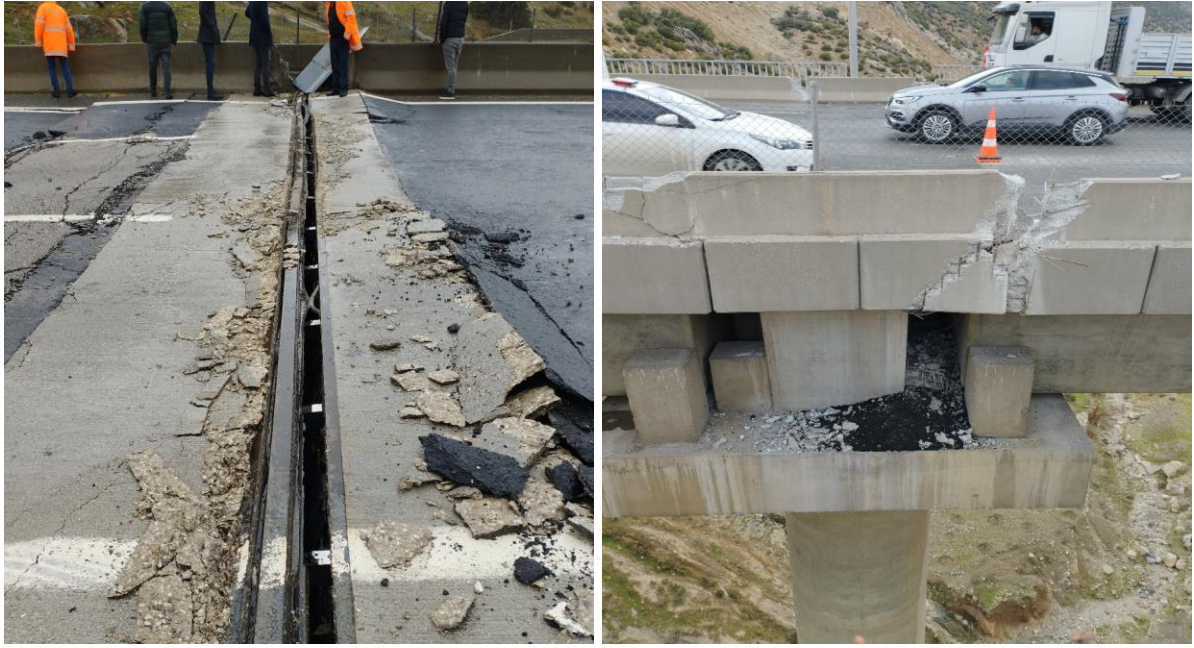
Figure 12. Damages on the Başpınar Viaduct
