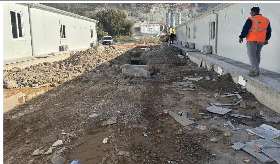
Figure 66. Non-Conformity in Kuruyer Construction and Accommodation Area
