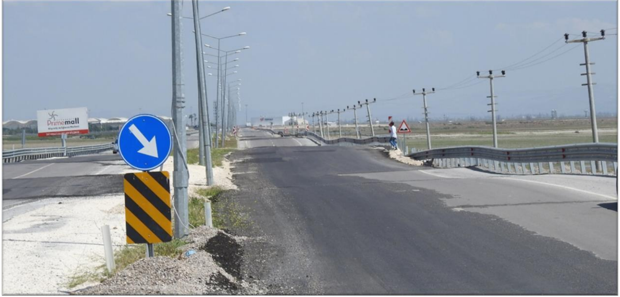
Figure 7. View of the Hatay Airport Road After the Earthquake (Km:2+840-3+480)
