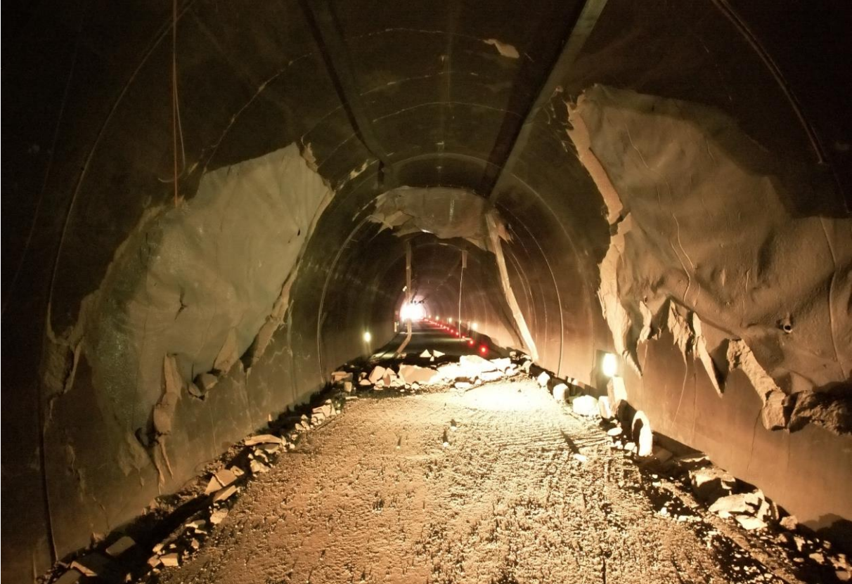
Figure 18. Damage on Erkenek Tunnel Entrance Portal Area
