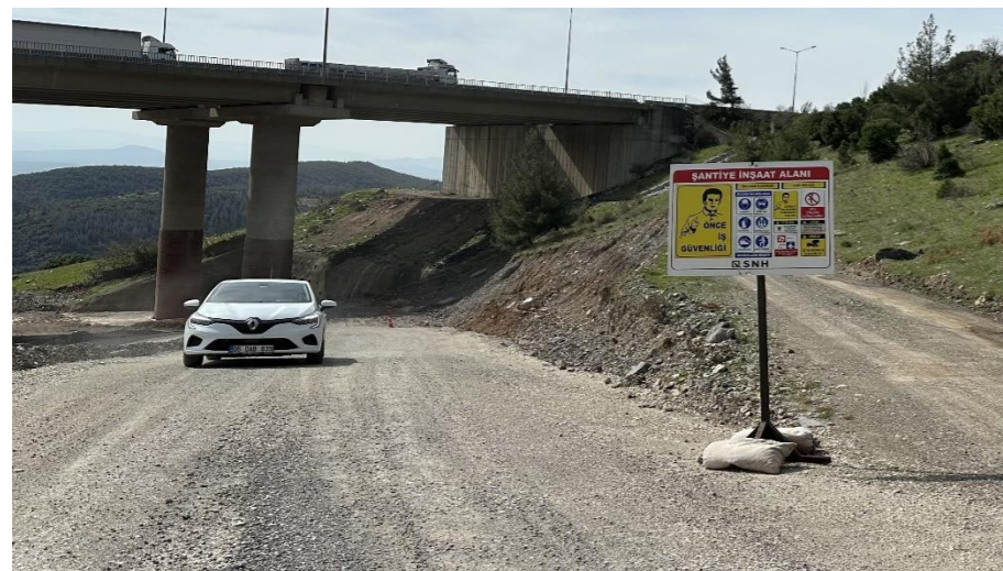
Figure 93. Information and warning signs in the activity area of Başpınar Viaduct
