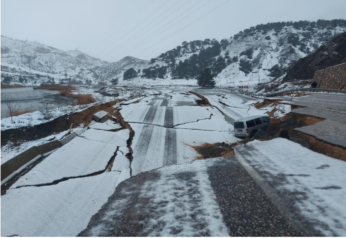
Figure 17. Damage on the Transformers Zone (Malatya-Gölbasi Road KM:89+260-KM:30+100)
