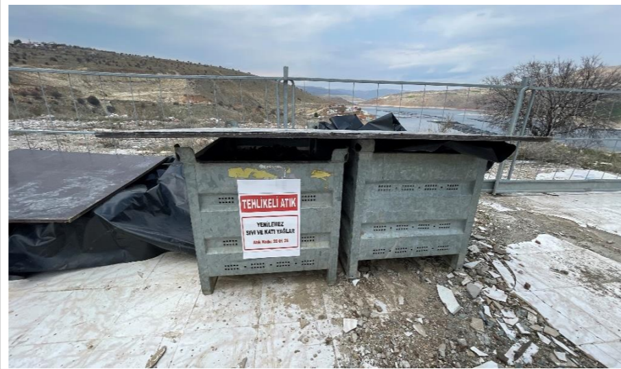
Figure 111. Hazardous Waste Containers in the Ağın Construction Site
