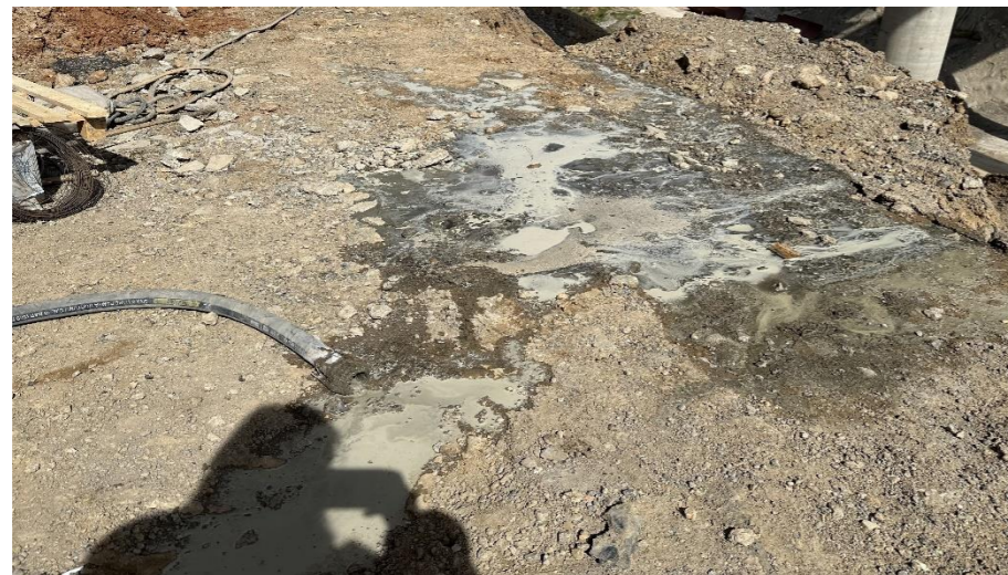
Figure 90. Soil Contamination in the activity area of Başpınar Viaduct
