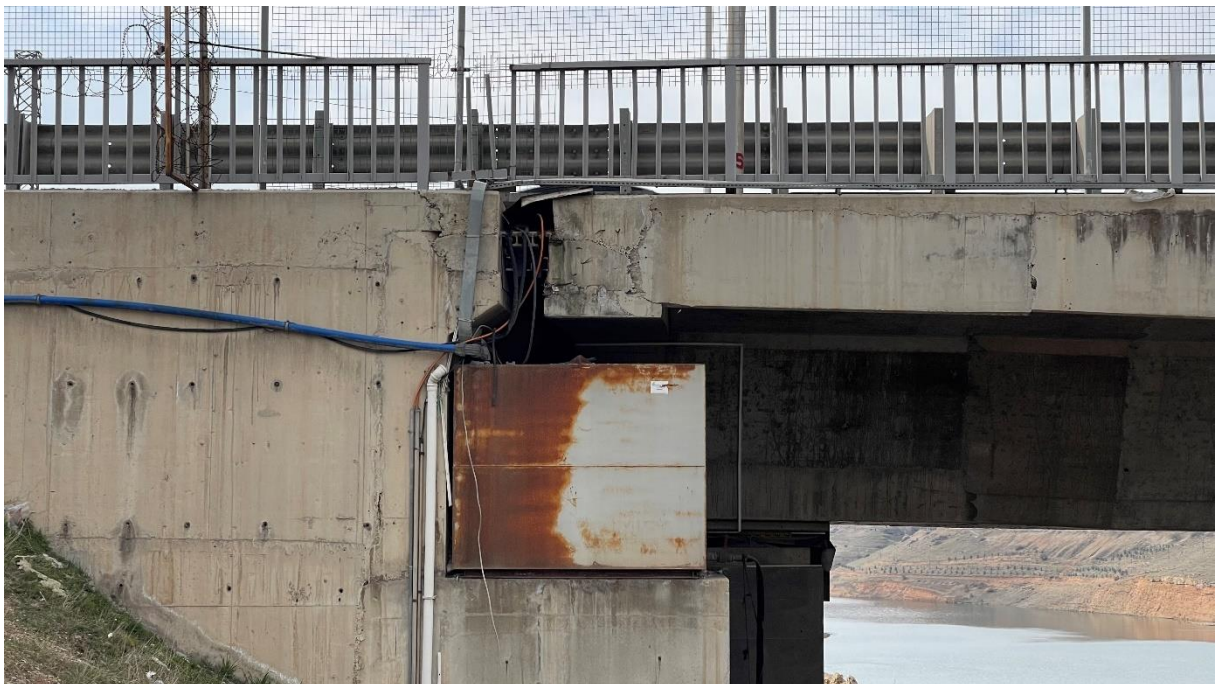
Figure 103. Damages on the Bridge
