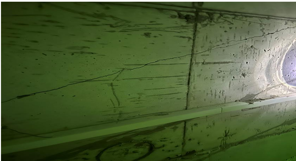
Figure 22. Hairline Shear Cracks
