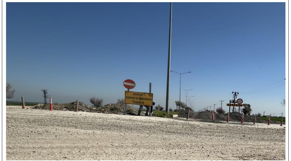
Figure 47. Warning Sign at the Hatay Airport Road Construction Site
