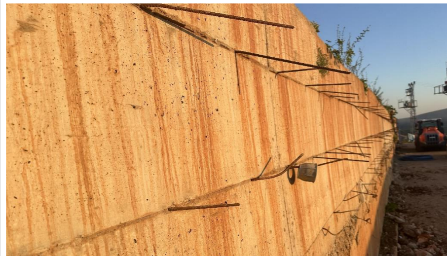
Figure 49. Non-conformity at the Kızılkaya Construction and Accommodation Site-1
