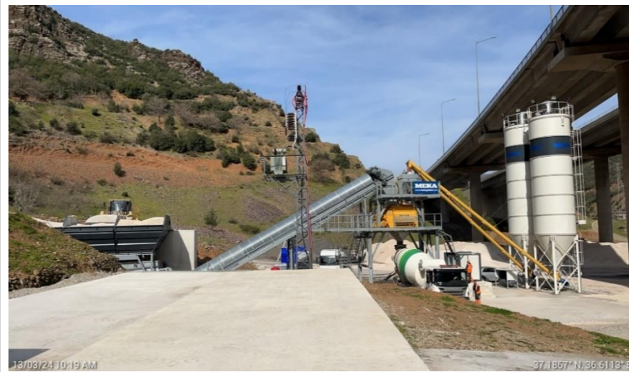
Figure 79. Bahçe (Ayrın) Concrete Plant
