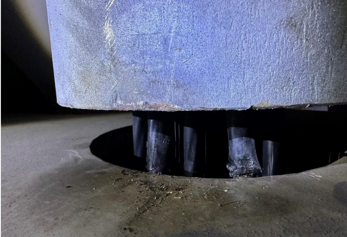
Figure 28. Damaged Suspension Cables
