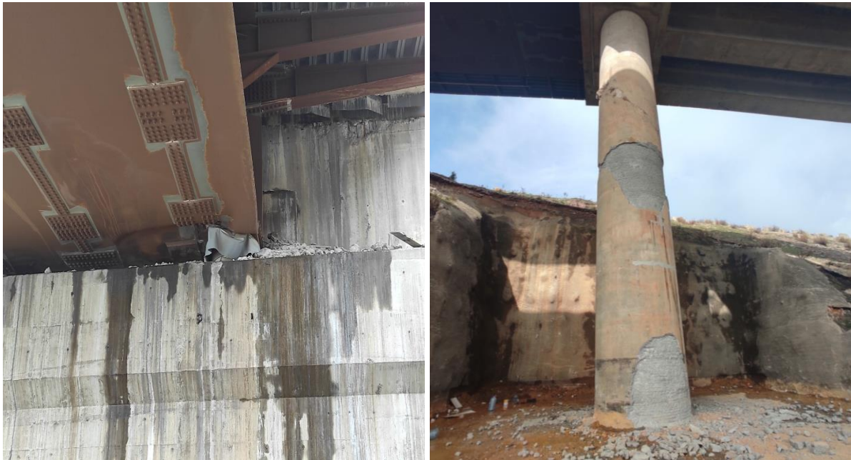
Figure 11. Damages on the Nurdağı Viaduct
