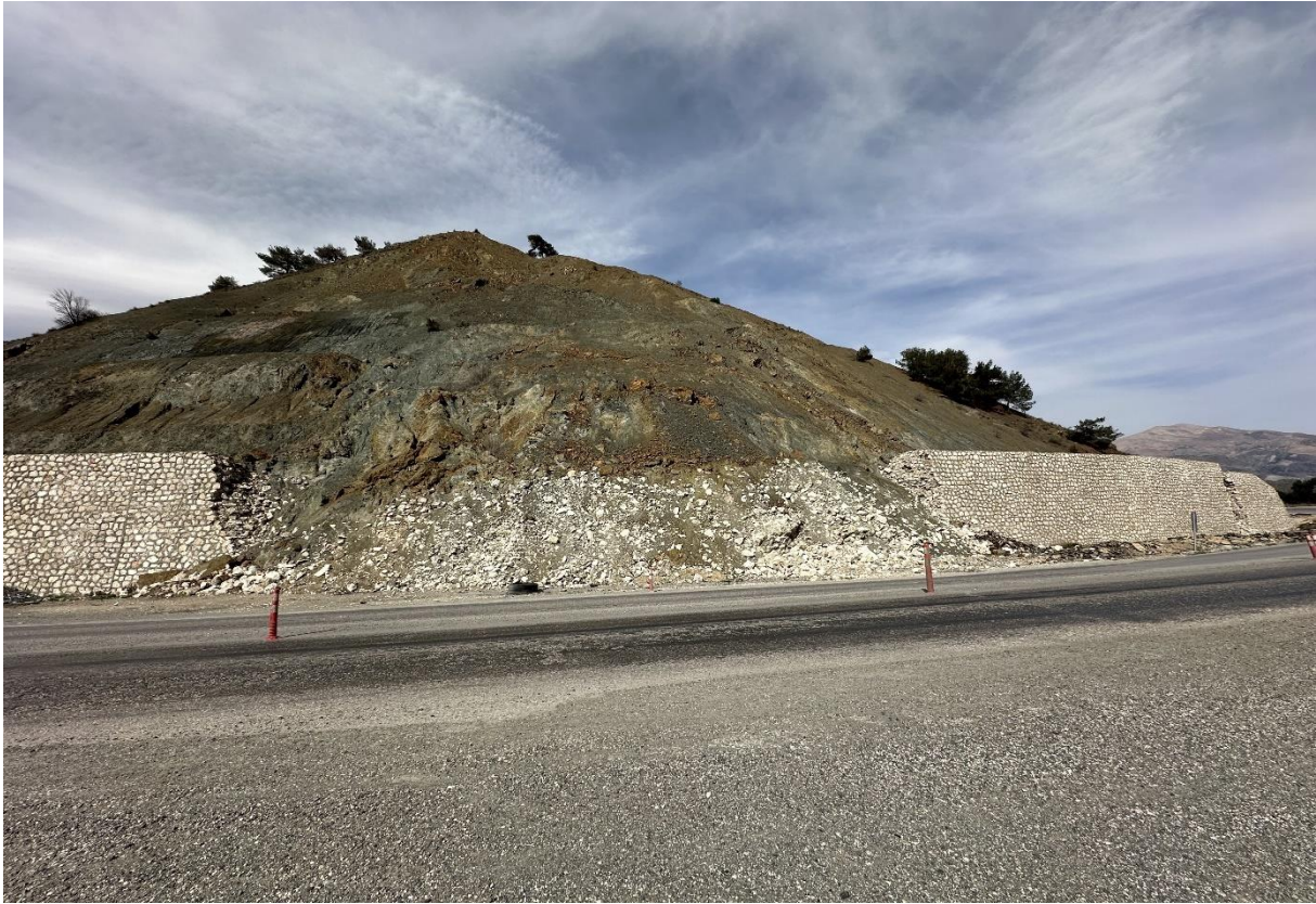
Figure 97. Damage on the Road – 2
