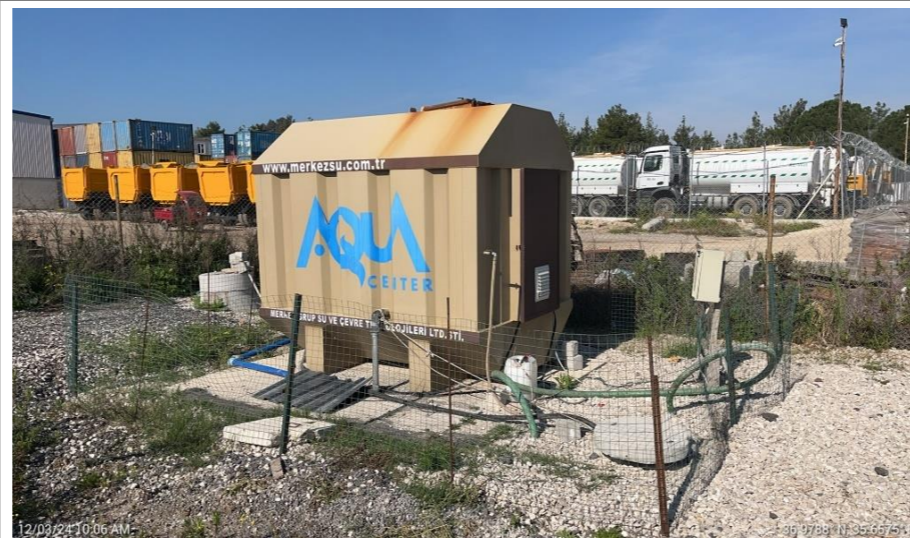
Figure 82. Package WWTP in Ceyhan Construction and Accommodation Site
