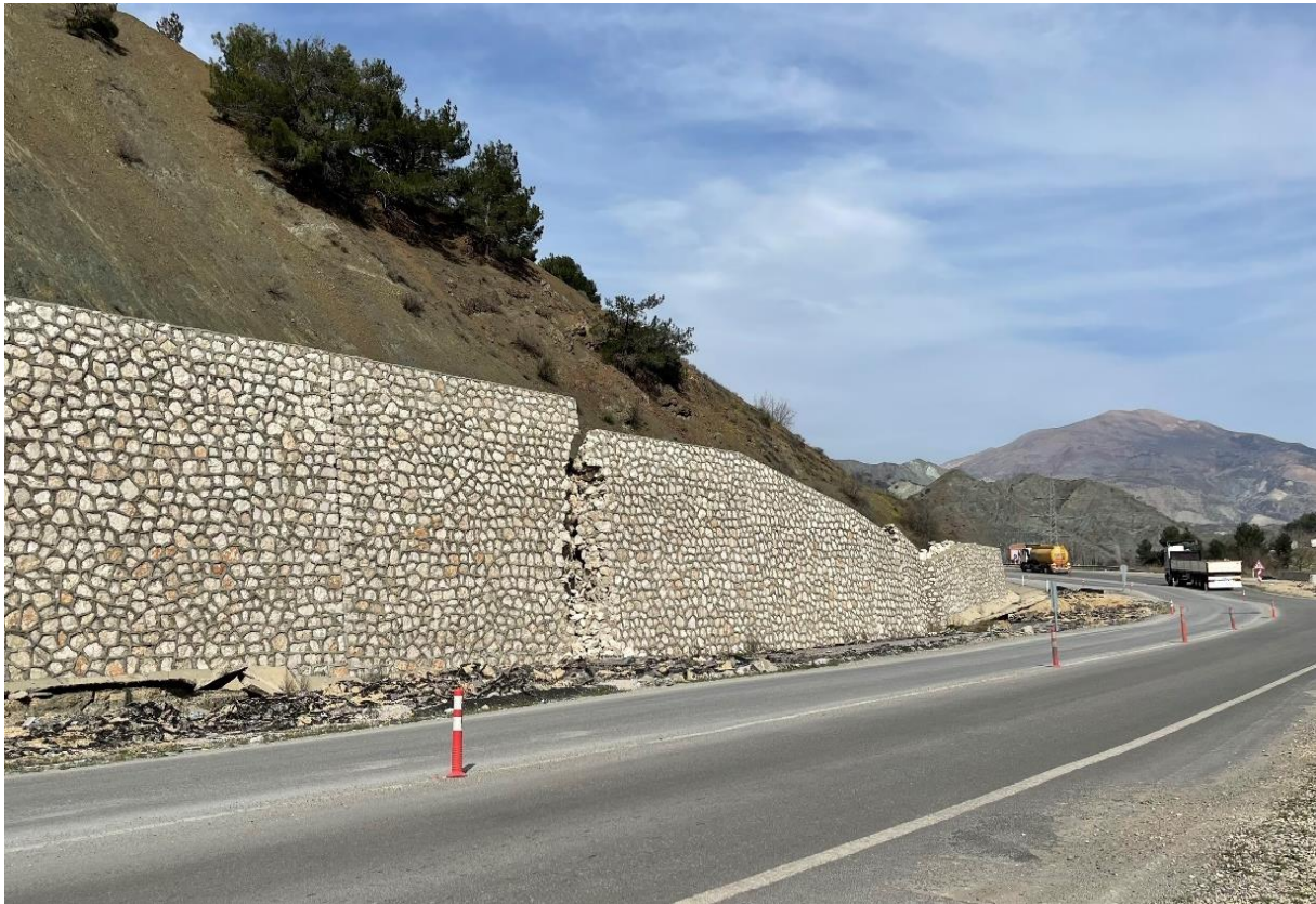
Figure 96. Damage on the Road - 1
