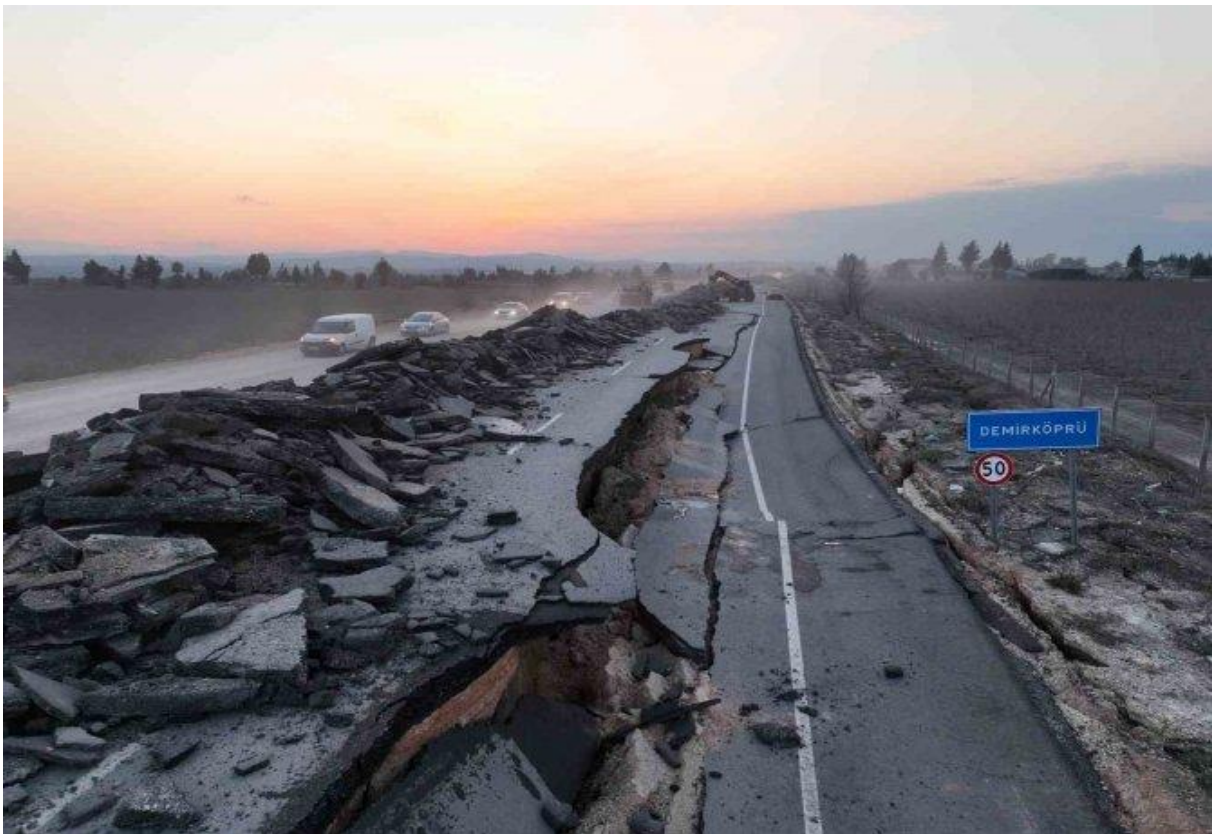
Figure 5. View of the Demirköprü Bridge After the Earthquake
