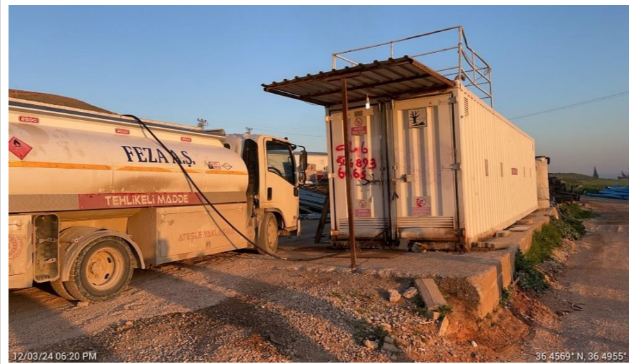
Figure 46. Chemical Storage Tank in the Kızılkaya Construction and Accommodation Site
