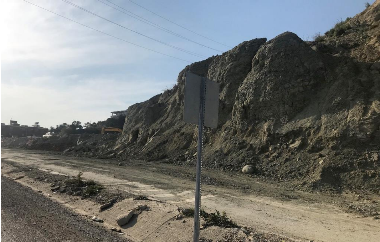
Figure 61. Landslide in Küçükkaracaay District Road
