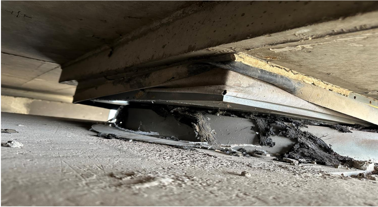
Figure 23. Damages on the Structural Bearings
