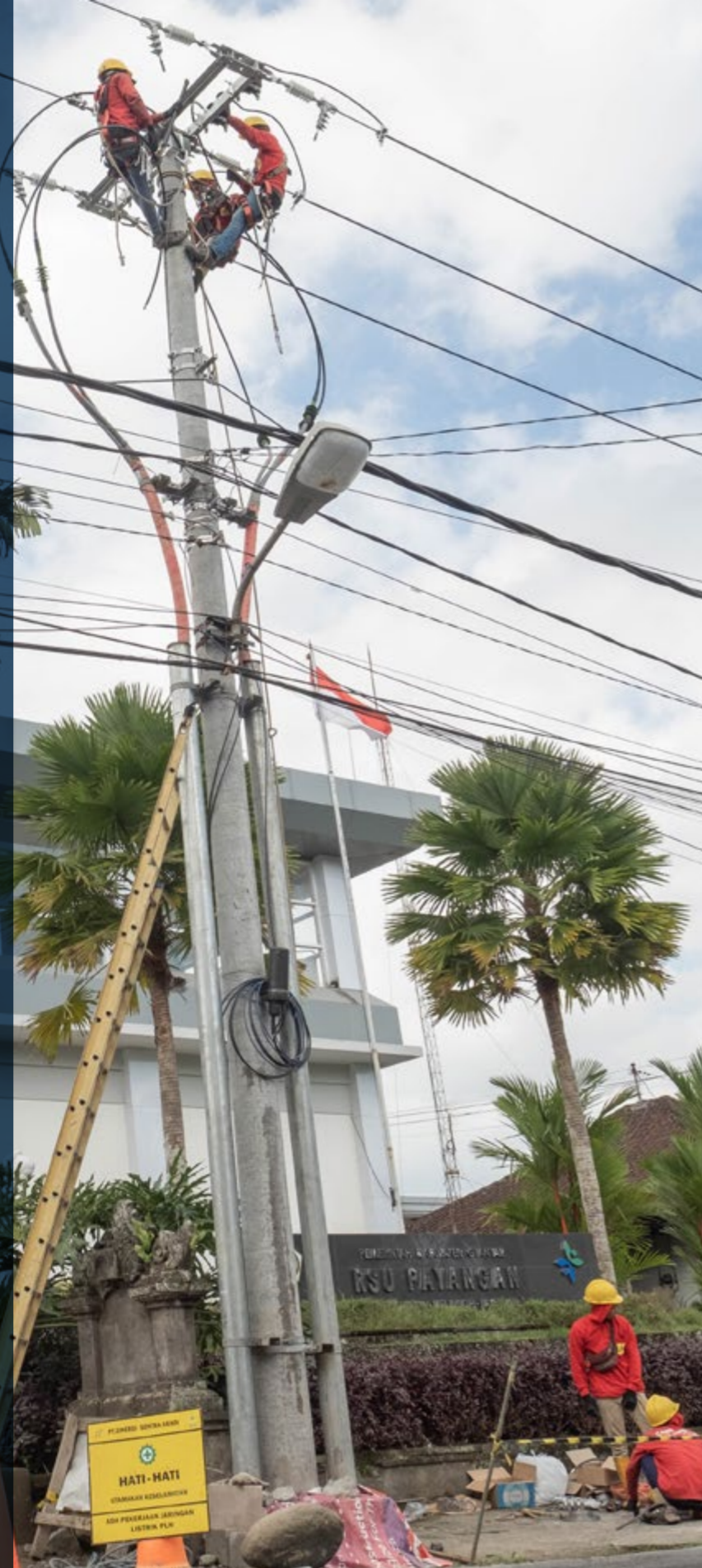
Indonesia & Bali Power Distribution Strengthening Project
